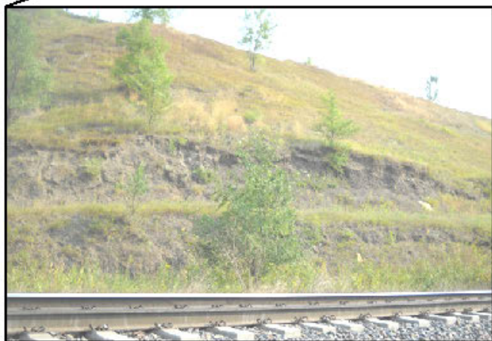
EXISTING EMBANKMENT DETERIORATION
