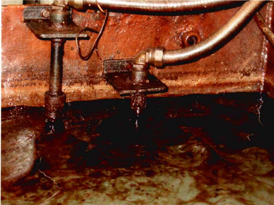
Oil in Condensate at the Hot Well – 5/2008
