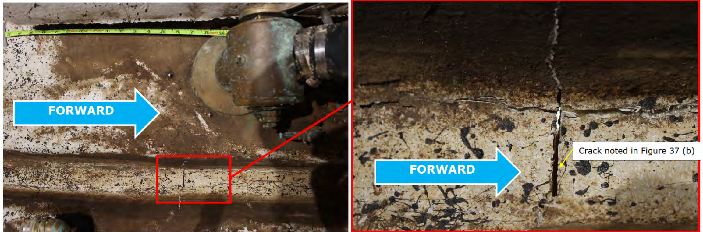
Figure 42. Photographs showing a transverse crack in the keel of the hull interior located 7.6 feet from the reference location. Tape measure is in feet.
