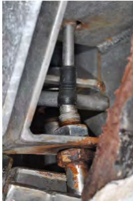
Figure 28. Photograph of the Subject Release Unit showing the as-found condition of the bulkhead nuts attaching the Subject Hydrostatic Cable to the Subject Release Unit.
