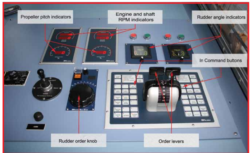
A vessel's engine control station features two identical arrays to control the two propellers. On either side of the order levers are 18 push buttons, 11 of which have assigned functions. These pushbuttons are identical in shape, color, and lettering, and each has a red LED in the upper left corner that illuminates according to functional status. The identical color, luminosity, and size may confuse users. Image courtesy of the United Kingdom's Department of Transportation Marine Accident Investigation Branch.
