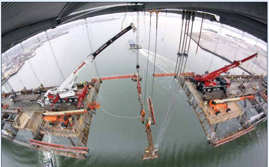
The fourth-longest steel arch bridge at the time of its completion in 1931, the Bayonne Bridge connects Bayonne, New Jersey, with Staten Island, New York. The process of raising the road bed from a height of 155 feet to deck to a height of 215 feet began in 2013 to accommodate New Panamax ships. The new road bed was opened to traffic in February 2017 and the process of removing the original deck began. Photo courtesy of Port Authority of New York and New Jersey
