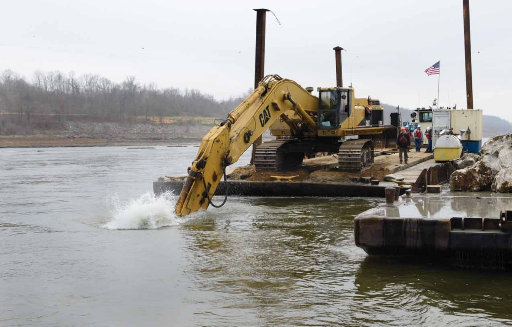
Workers contracted by the U.S. Army Corps of Engineers (USACE) clear rocks from the Mississippi River floor near Thebes, Illinois, in December 2012. The Coast Guard and USACE supervised these rock blasting operations in an effort to mitigate the low water situation on the Mississippi River. Coast Guard photo by Petty Officer 3rd Class Ryan Tippetts
