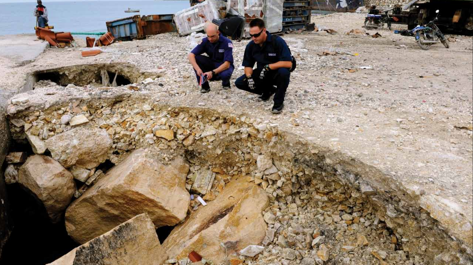
Coast Guard LCDR Eric Carrero, international port security liaison officer for Haiti, and LTJG Mike Clausen from the Coast Guard District Seven Marine Transport System Recovery Assist Team (MTSRAT), inspect a section of the pier that collapsed in November 2010 during Hurricane Tomas. The MTSRAT deployed to Haiti to conduct an assessment of the marine transportation system and the condition of the piers for vessels to dock and offload supplies. Coast Guard photo by Petty Officer 3rd Class Sabrina Elgammal
