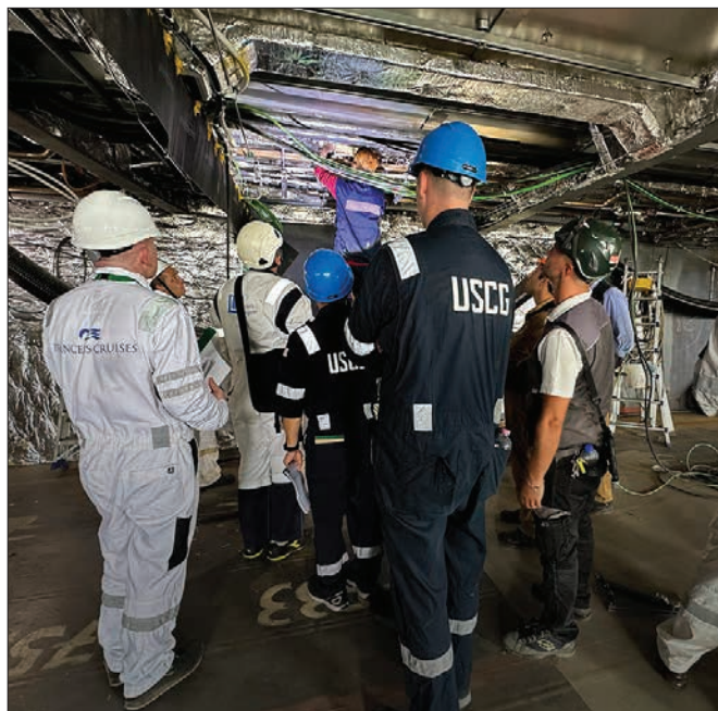
Coast Guard marine inspectors observe structural fire protection installation at the Monfalcone Shipyard in Trieste, Italy. Coast Guard photo by LT Sam Morrison
