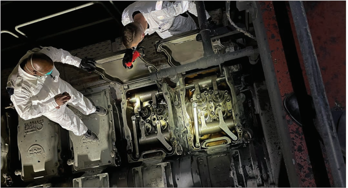
Coast Guard inspectors LT Todd Cooper and LT Tim Powell conduct an internal inspection of a ship's diesel generator following a fire. The picture is taken from the catwalk above the engine bay looking down at the exposed heads of the engine cylinders. Coast Guard photo by LCDR Walter Hutchins
