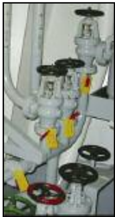
Seals and tags for overboard lines and flanges prevent unauthorized engineering changes.
