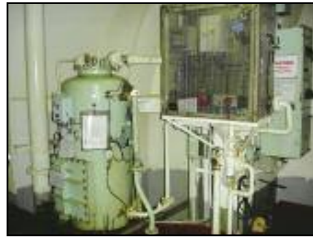
Oily water separator oil content meter.
